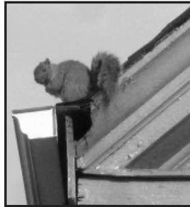
deteriorating in some places.
